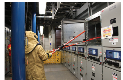
Dressed in protective suits, electricians are confirming voltage levels (phase and rotation) across an electrical breaker at GMS. Through these Station Service Panels, power is provided to the GMS Powerhouse.
