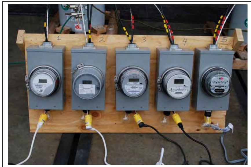
Figure 2 – Meters Subjected to the Over-Voltage Tests
