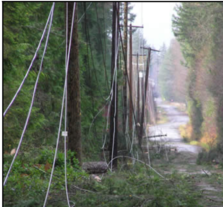
BC Hydro plans to enhance the resiliency of the most vulnerable portions of the distribution system.
