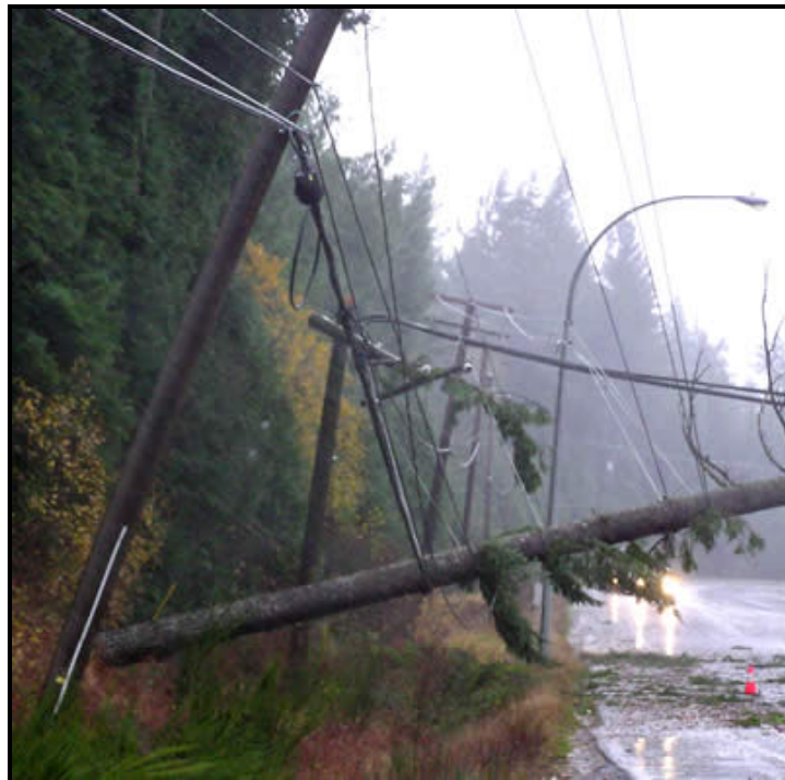
BC Hydro plans to identify and prioritize for removal trees that have a high potential to damage the distribution system.
