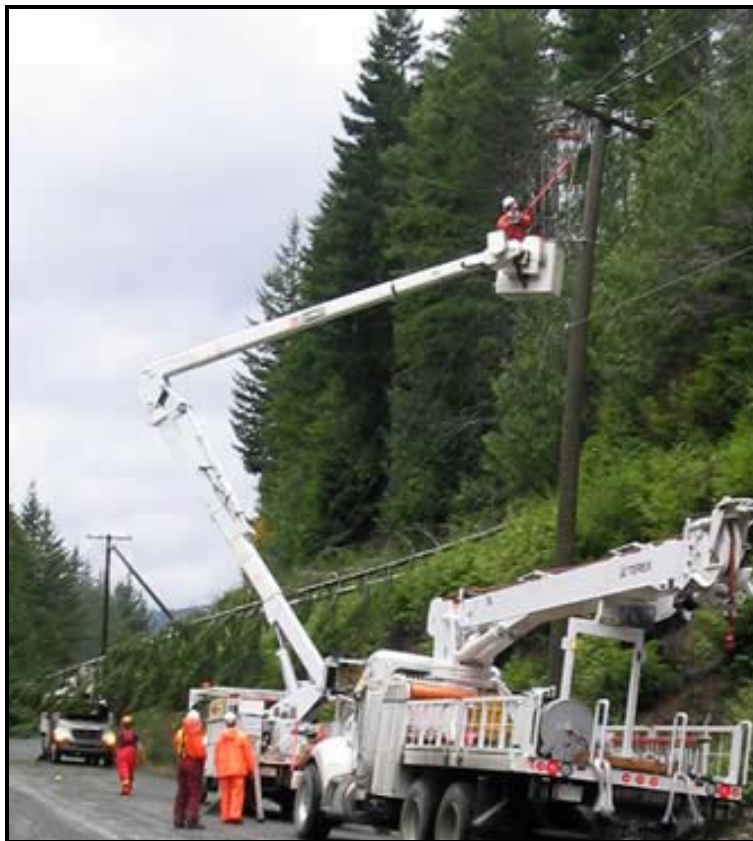
Nearly 500 employees were directly involved in the restoration effort at the peak of each storm, including as many as 188 power line technicians.
