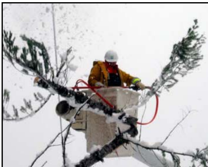
In Northern B.C., heavy, wet snow toppled trees and limbs onto distribution lines.
