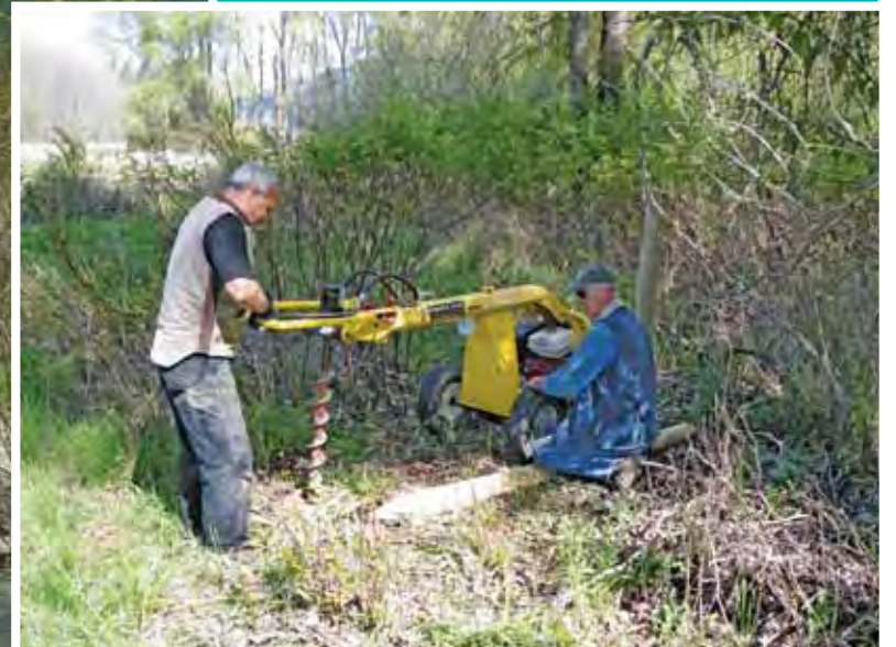
Volunteers from the Creston Valley Rod and Gun Club bore holes for the fence posts.
