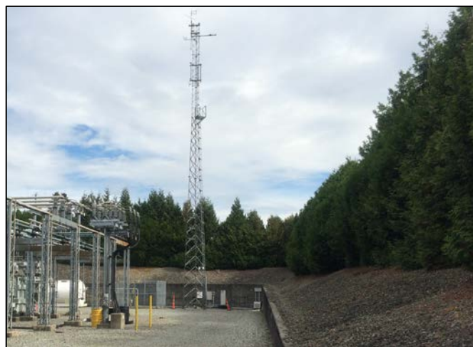
Existing telecommunication tower at Mainwaring Substation
