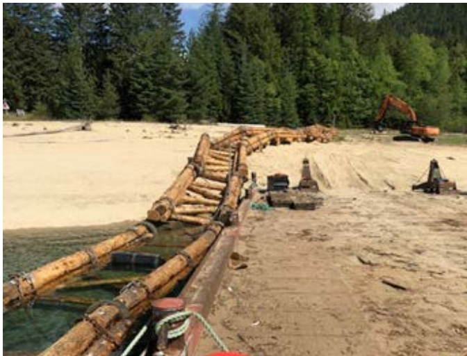
The new north breakwater at the MacDonald boat launch. Credit: Brooklyn Barge & Tug.
