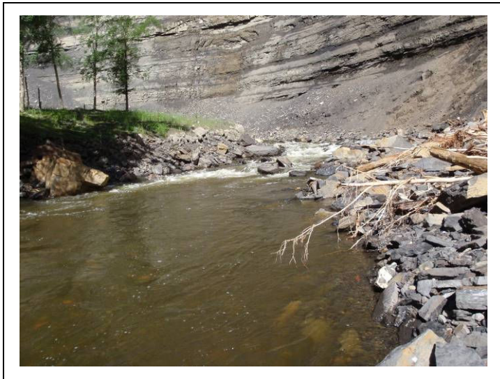
Plate 39. Upstream view of the channel on Gething Creek, 430 m upstream of the reservoir.
