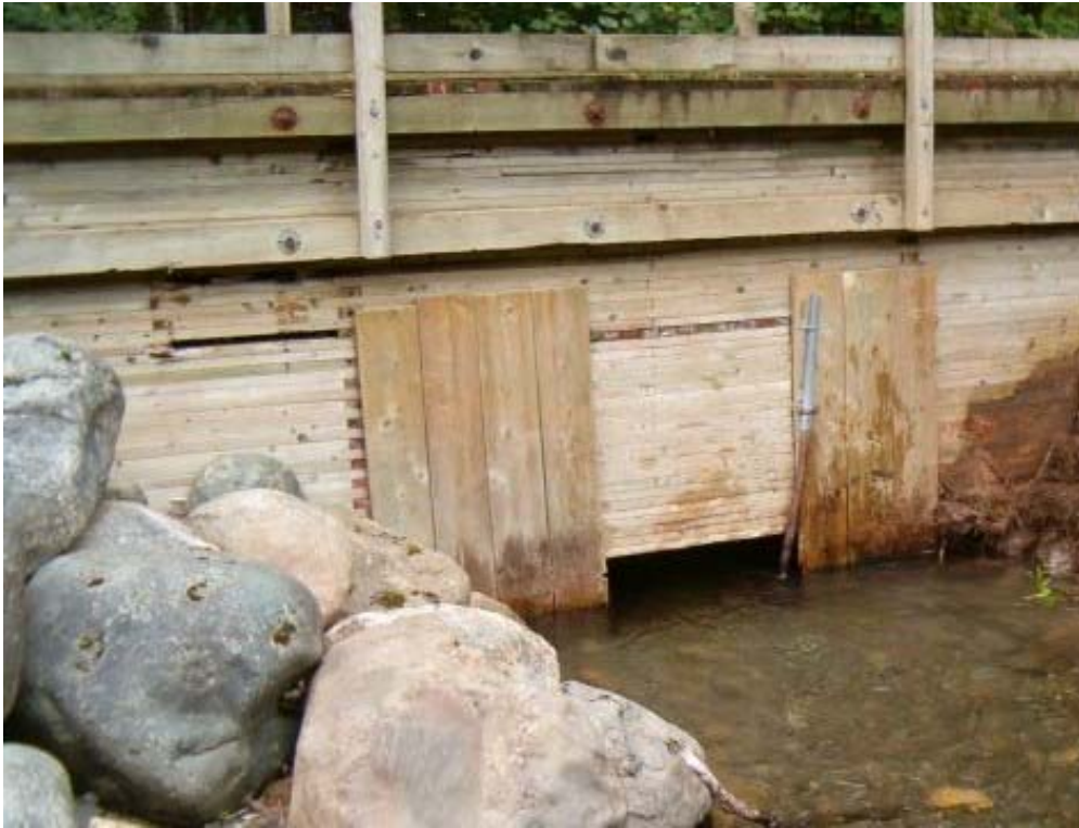
Figure 3. Inlet channel and footbridge providing flow control to the Powerhouse side-channel before installation of pipeline.
