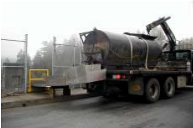
Carcass distribution Tank-truck
