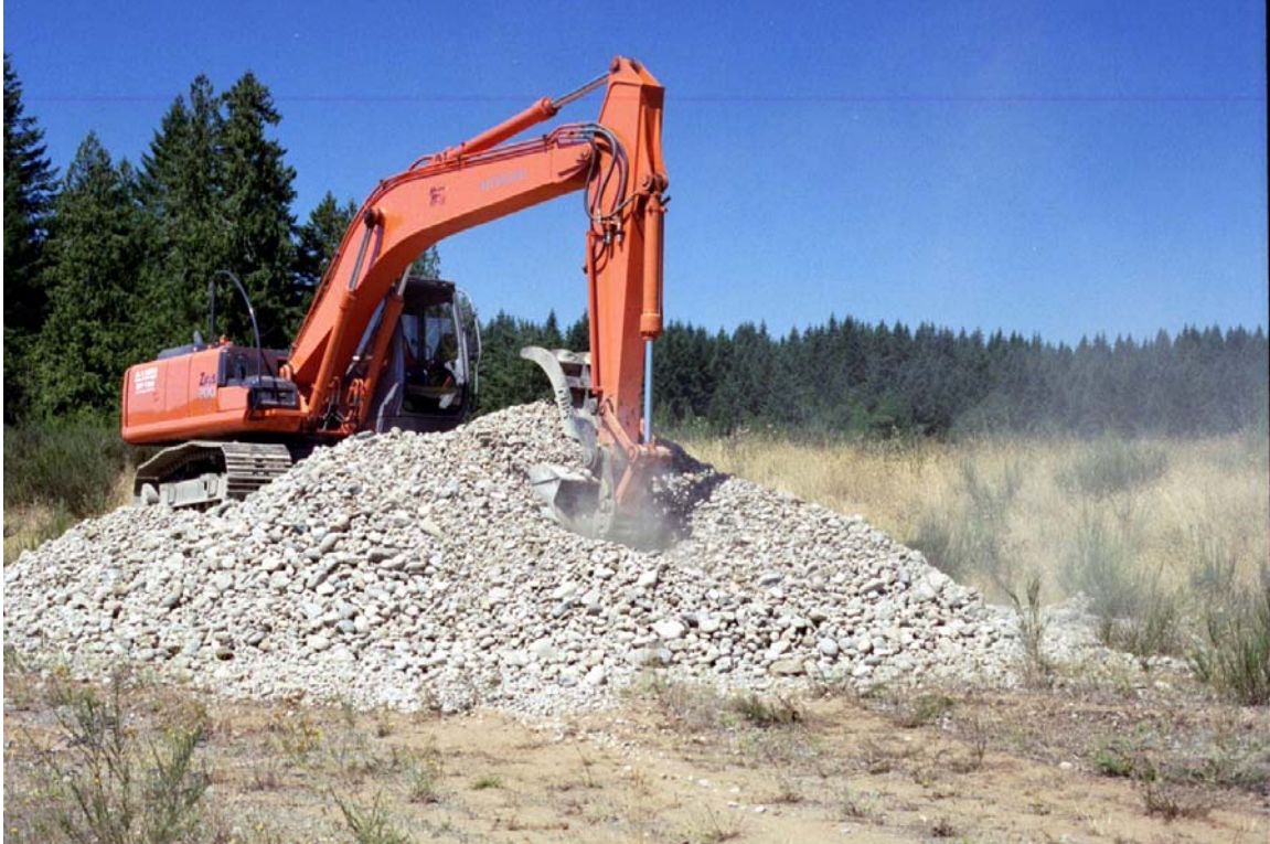
Photo 3. An excavator was employed to mix and load the gravel substrate into buckets. Virtually all of the substrate was delivered into two sites.
