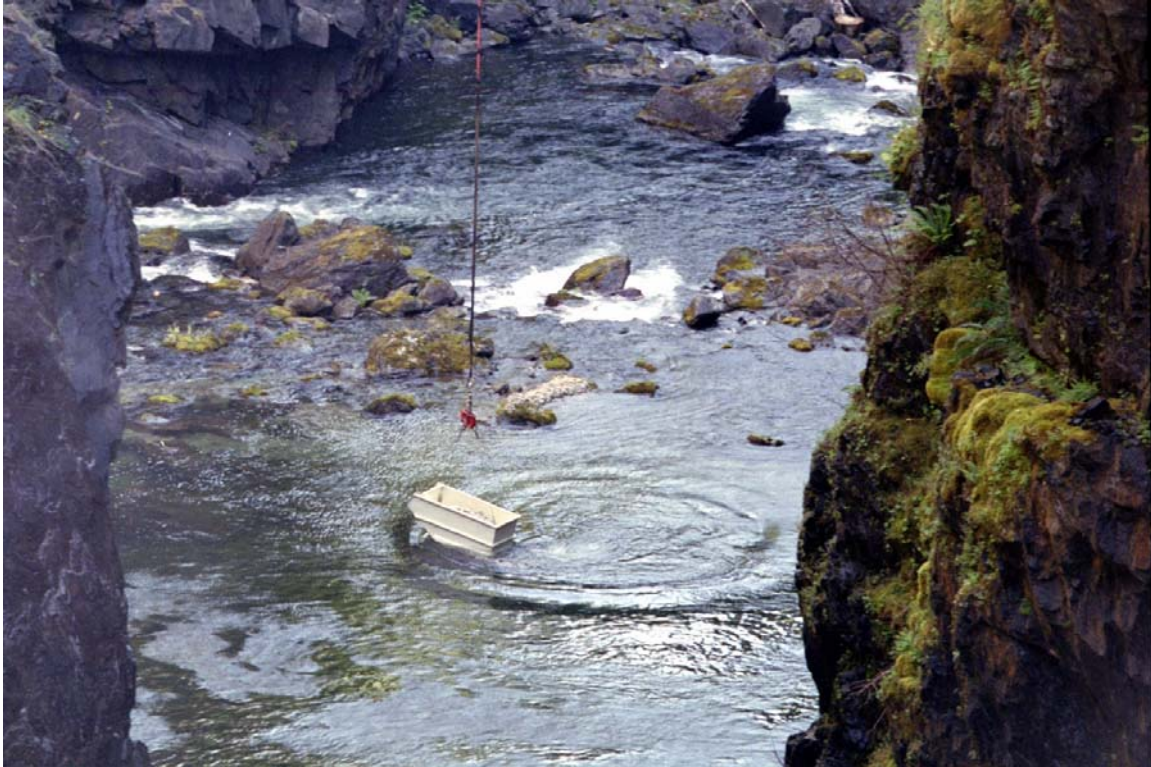
Photo 5. Placing gravel in the tailout of the Elk Falls plunge pool. Note: gravel bucket has not been remotely dumped at the time of photo.
