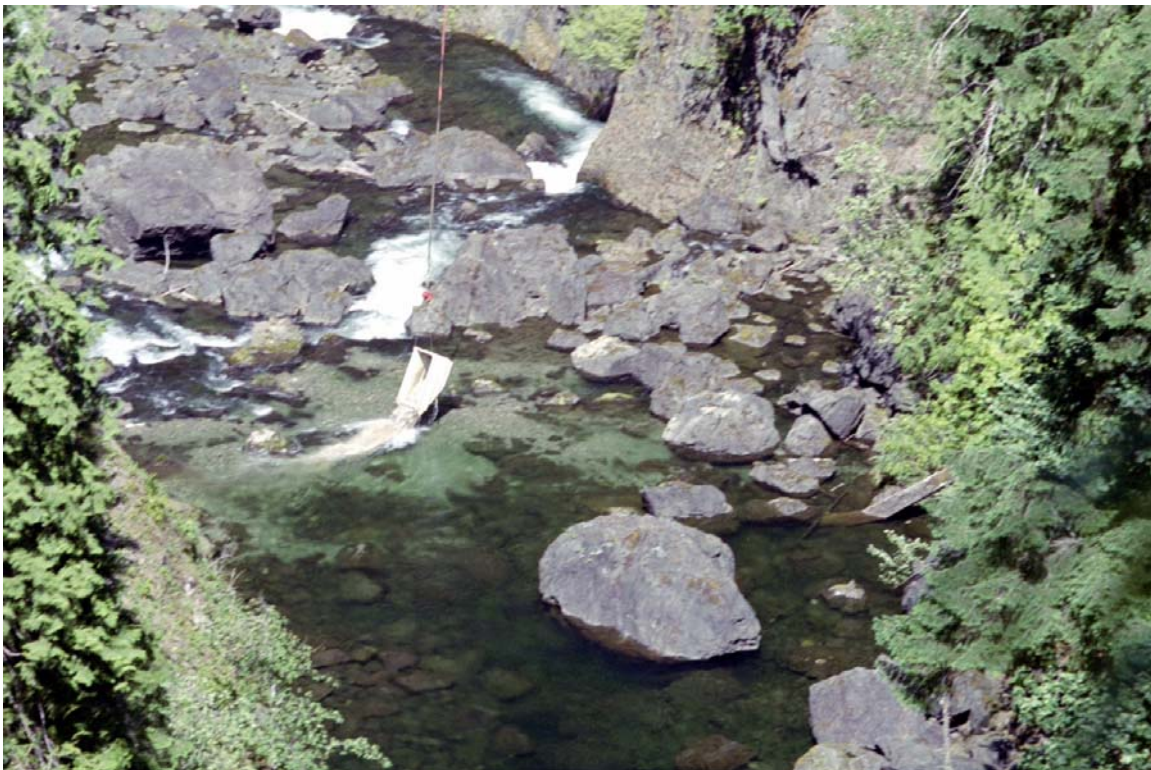
Photo 6. Placing gravel in the lower (primary) location. Note: The gravel bucket has been remotely released and substrate is spread laterally across the tailout.
