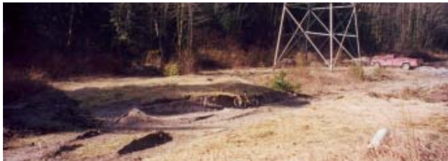
Figure 4. The site around the base of the transmission tower early in construction.
