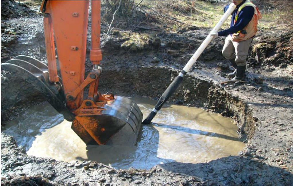
Figure 5: The monitoring wells were made of 3.05 m lengths of 10.2 cm perforated plastic pipe that was wrapped with filter cloth. They were buried about 2.8 m below ground level with 0.2 m of pipe exposed above ground.
