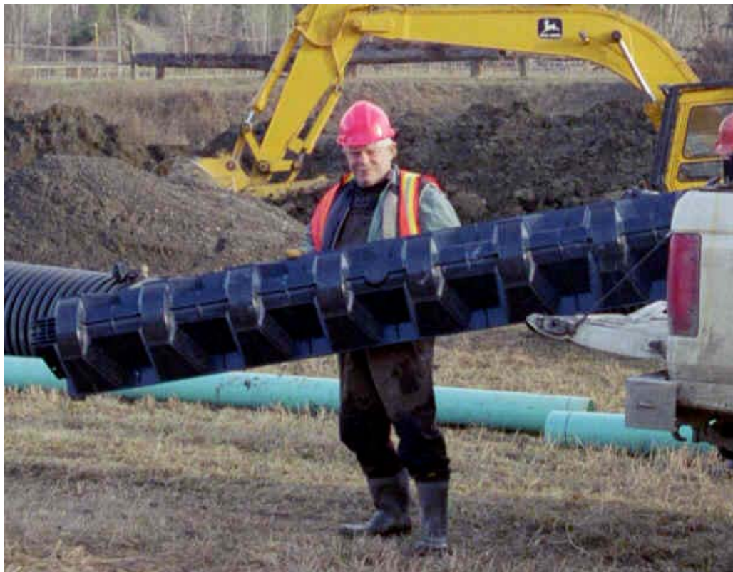
Figure 12: Worker holding a section of infiltration gallery. The infiltration galleries are shaped like an inverted “V” with an open bottom. The sides have fine louvered openings so that they are permeable to water but resist filling with sand (Figure 12). They have been used successfully by DFO and WCRC on several projects.
