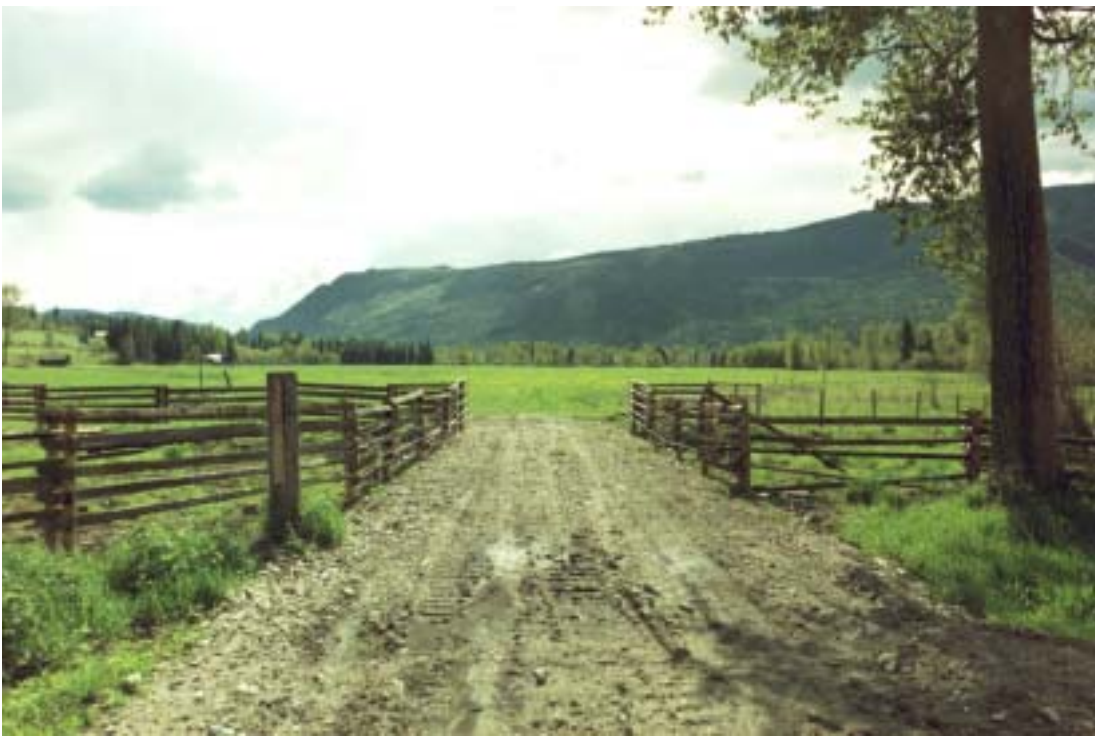
After 16: This tributary crossing on the 459218BC Ltd property after a culvert and gravel were placed and the fence rebuilt.
