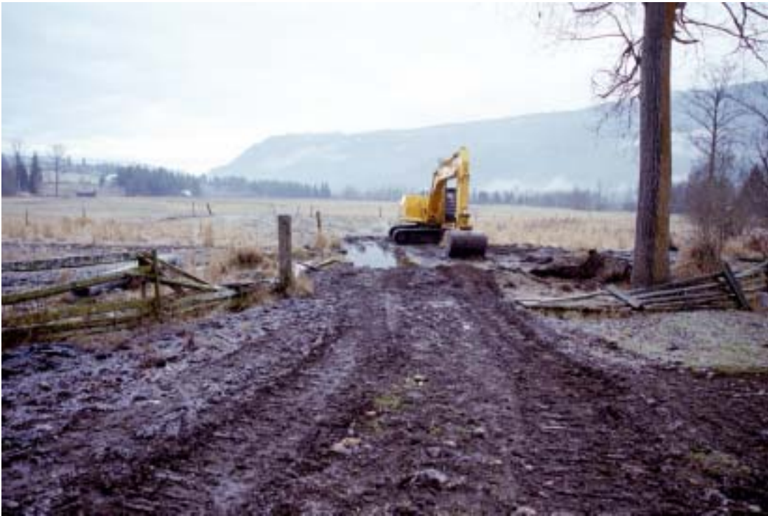
Before 16: The old culvert had been plugged from trampling by cattle making this crossing unusable most of the year.
