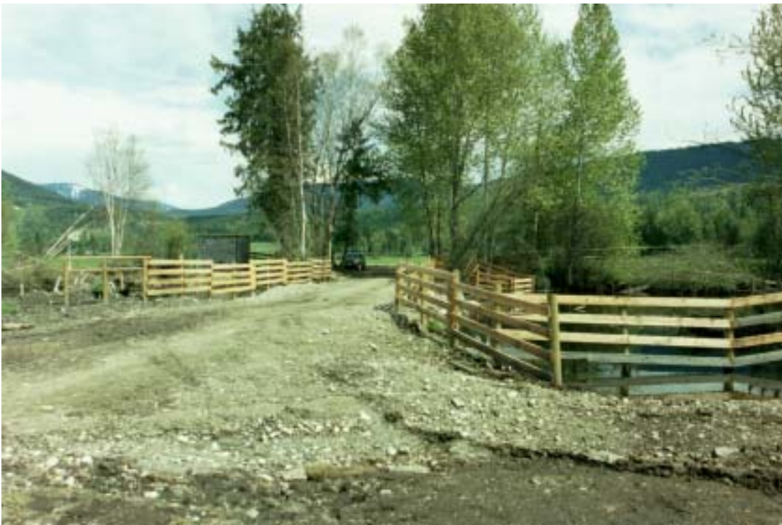
After 11: Culverts have been added and the crossing graveled and fenced. There are cattle access points on both sides of the crossing.
