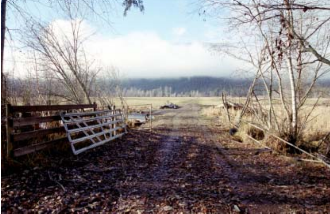
Before 10: The Chambers crossing looking westward. There were no functioning culverts before construction.
