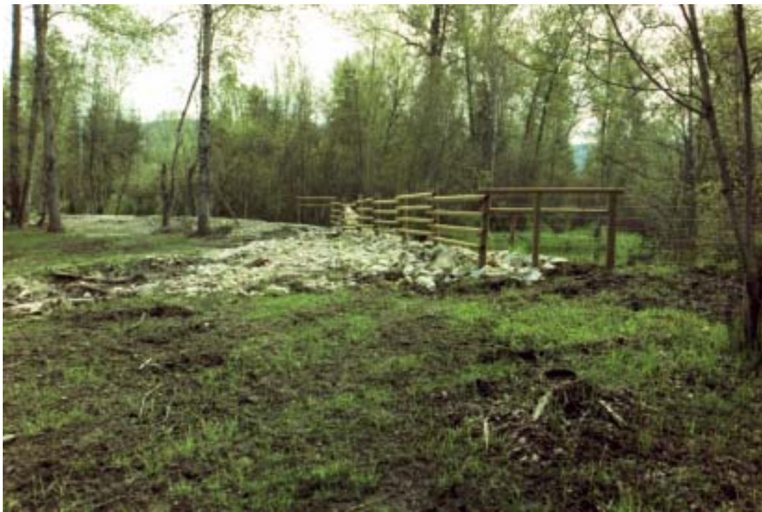
After 30: The same view as above with the corner rounded and armoured and the hole filled.
