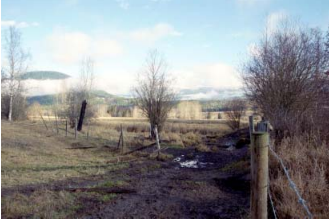
Before 15: The old culvert had washed out and the crossing had been trampled to the point that it was no longer usable. This is the southernmost crossing on the property owned by the 459218BC Ltd.
