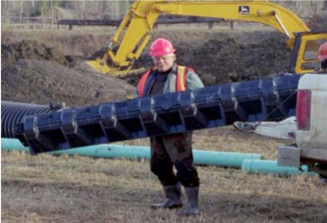
Figure 5: Larry McGregor holds up a section of the intake gallery. The sides have slots that angle downwards. Water is able to flow in, but sand and gravel is kept out. This type of gallery has a larger exchange area than standard perforated pipe.
