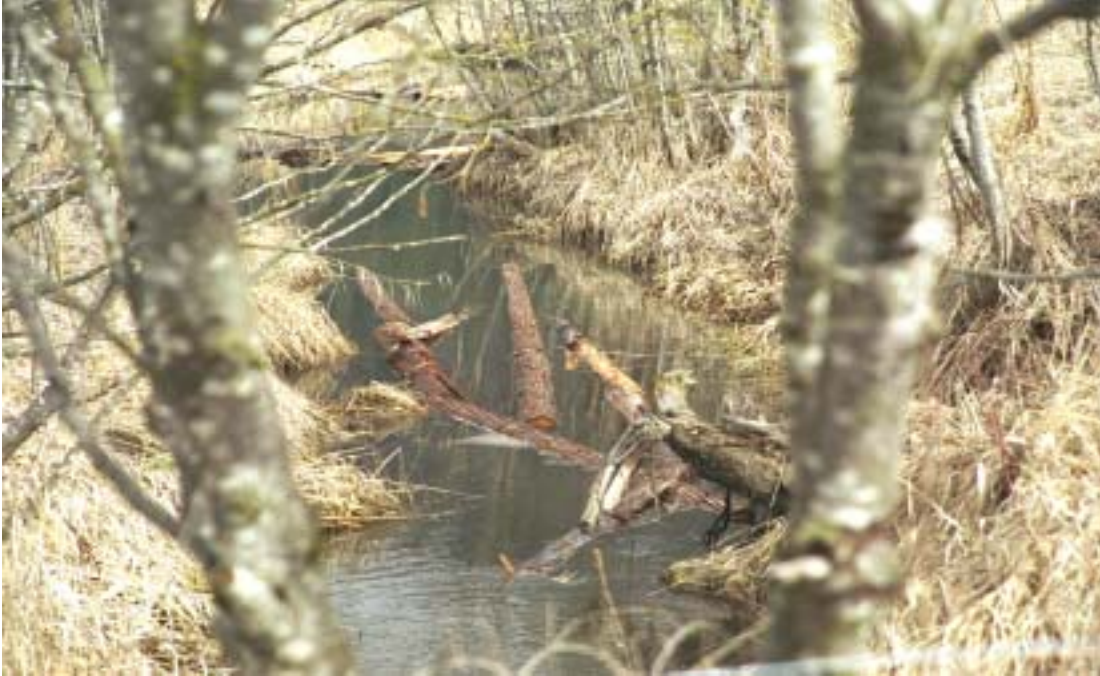
Figure 8: The slabs were chained together and anchored to the bank in various configurations to give them a random appearance. This method allowed the placement of woody debris in areas where there were not machine accessible. There is very little disturbance of either the riparian area or the stream using this method.
