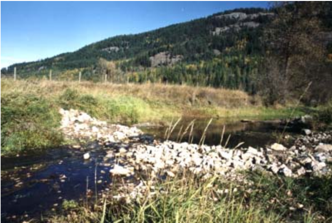
Figure 16: A riffle was built on the lower end of the channel to raise the water level by 30 cm. The creek and water table levels were the lowest the landowner (since 1970) had seen them. Placing the weir at the intake to increase the flow to the side channel and building the riffle on the lower end increased habitat values.
