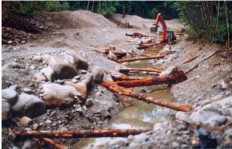
Figure 17. The groundwater channel nearly completed with wood and rock. The groundwater is half a foot deep (September, 2002).
