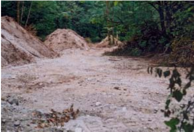
Figure 2. North end of site looking south to north pond after clearing brush and soil
