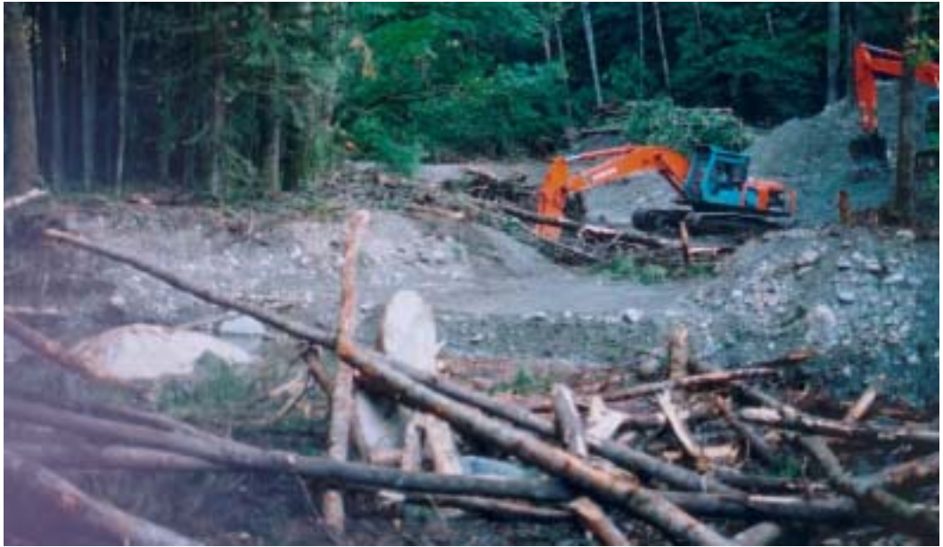
Figure 8. Excavators dig the deep portions of the north end of the north pond, as seen from south edge of the north pond.
