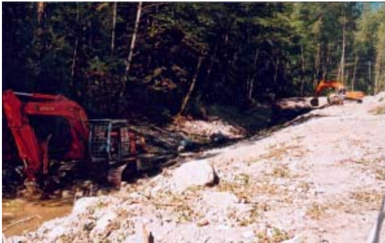
Figure10. Excavators dig the groundwater channel. Foreground machine is digging final grade and background machine digs the second pass to finish the width of the full channel and grading.
