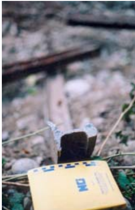
Figures 19 to 21. The rail segment we removed was 12 feet long and we broke it to remove it. The rail was three feet below ground, probably buried during the flooding of the mid 1950s.
