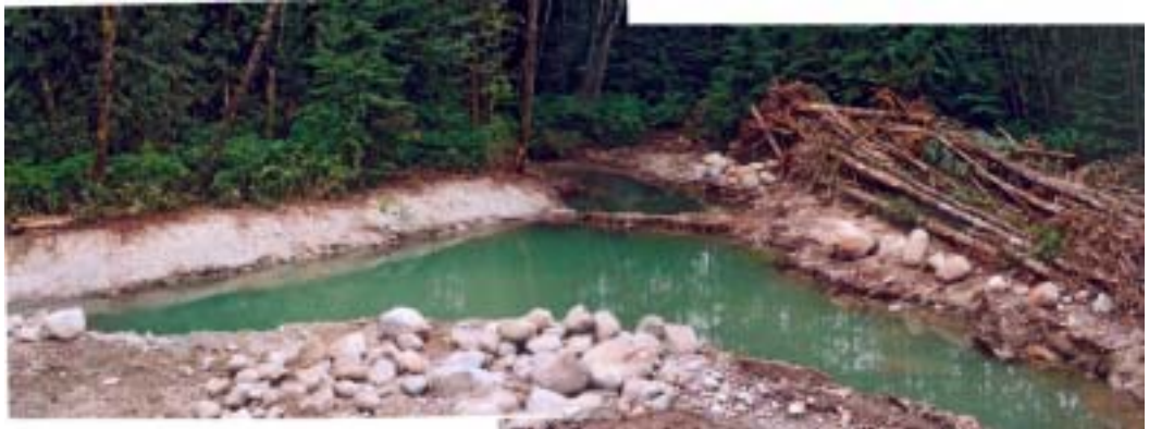
Figure 3 & 4. South Pond during construction showing separation berm after settling over night (3) and during construction (4)
