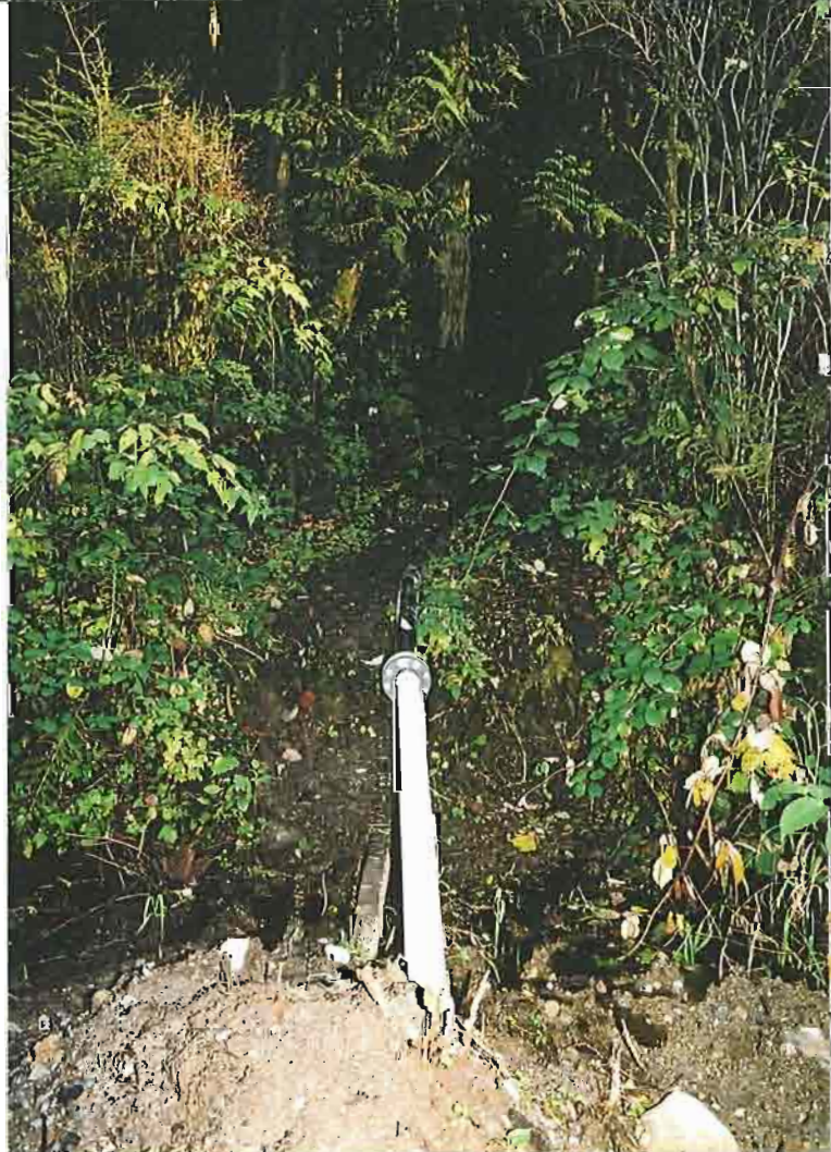
Photo 6: Connection to manifold trunk line.
