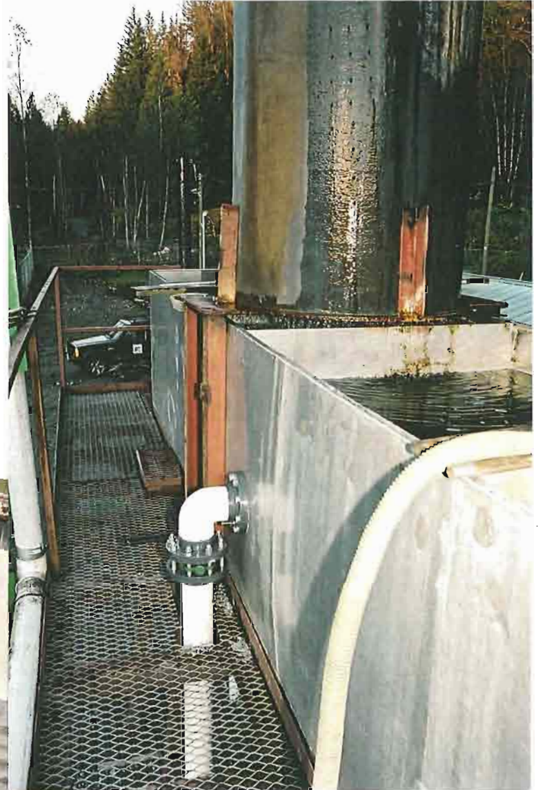
Photo 7: Head tank at upper hatchery illustrating 4" pipe line leading to lower hatchery cross- connect.
