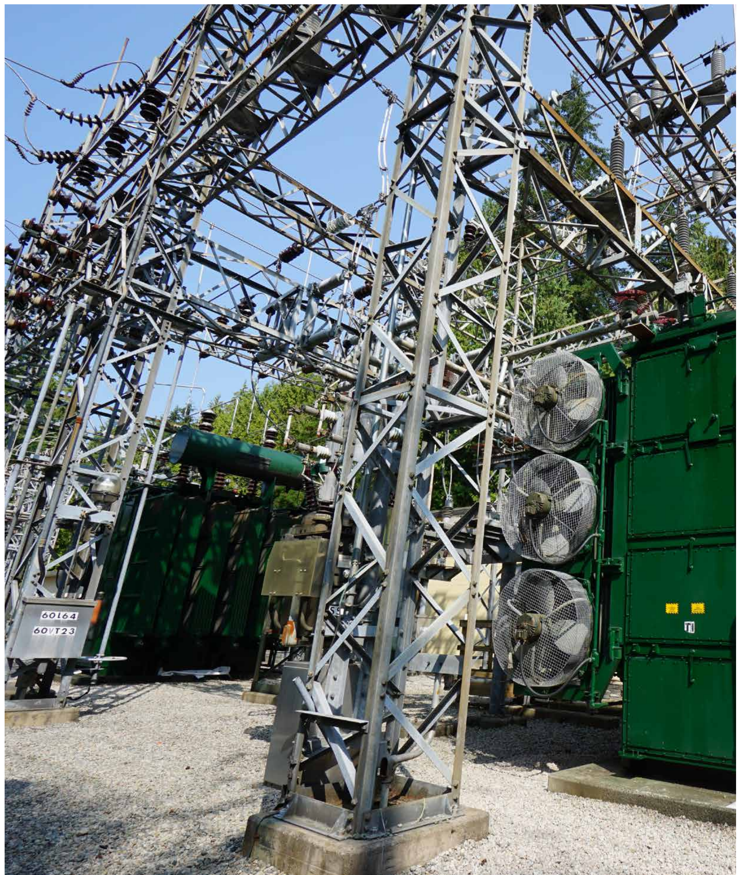
Existing substation inside the fence
