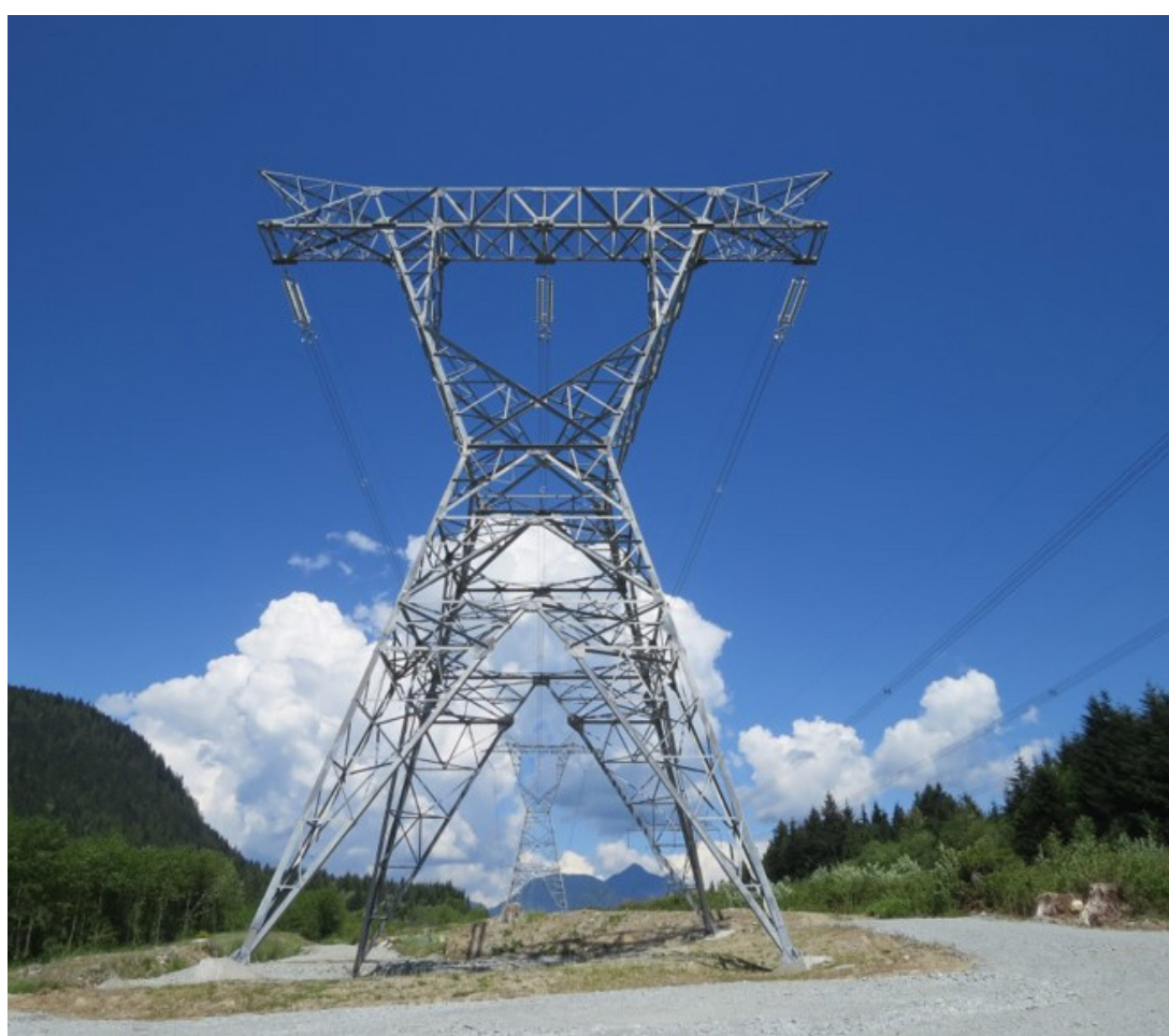
500kV Self Support Lattice Dead-End
