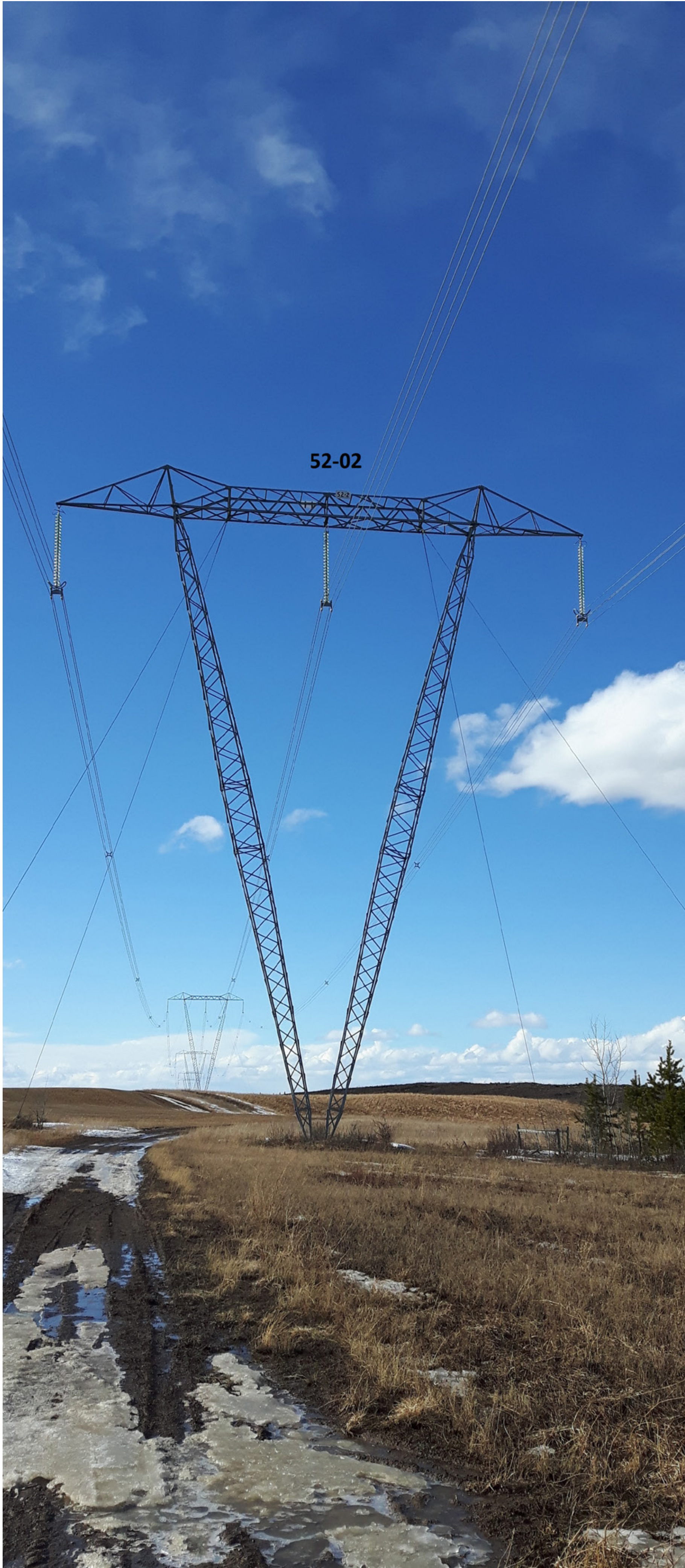
Existing 500kV transmission line
