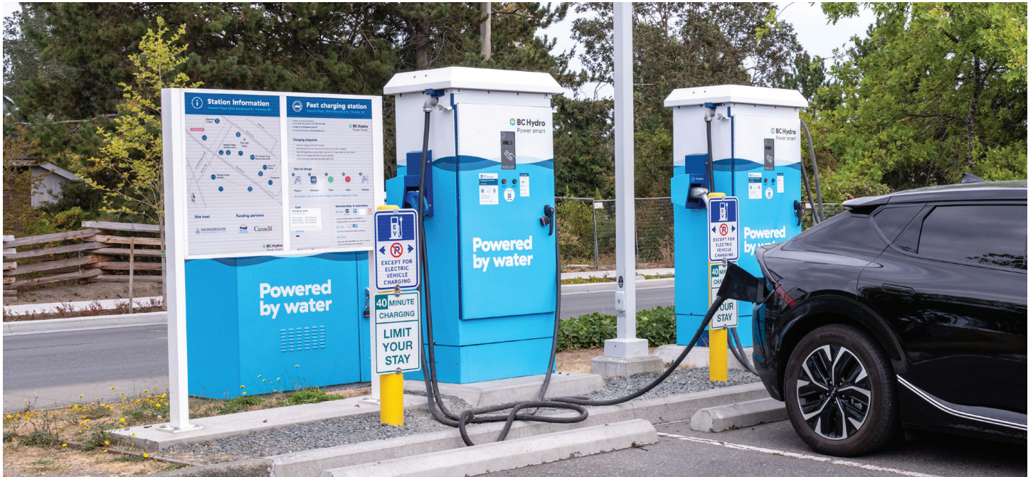
Figure 3: BC Hydro side-by-side informational signage at an EV charging station
