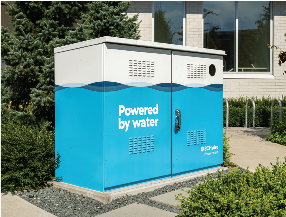
Figure 1: BC Hydro kiosk for EV charging station
