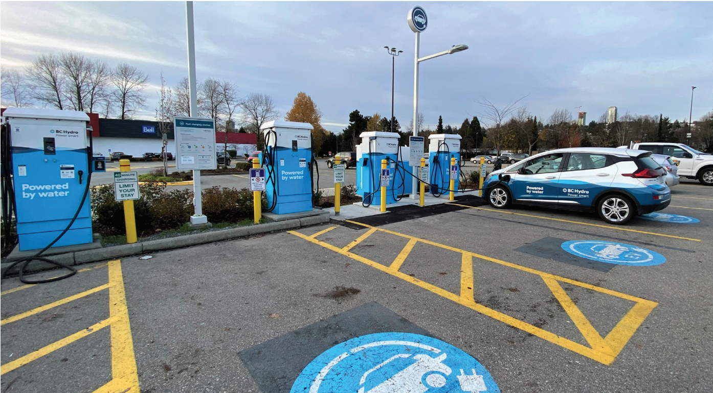
EXAMPLE OF A BC HYDRO STATION, PULL-IN, CHARGERS IN FRONT OF STALL
