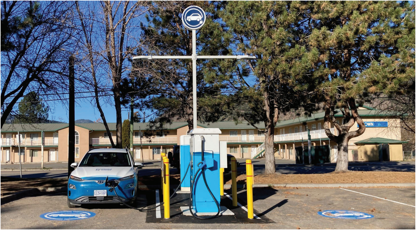
EXAMPLE OF A BC HYDRO STATION, PULL-IN, CHARGERS BETWEEN STALLS
