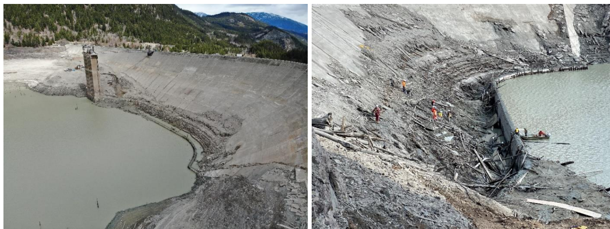
Figure 10 La Joie Dam during the spring 2022 drawdown. Note the significant volume of debris located on the toe of the dam.
