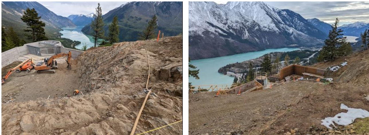
Figure 8 Construction of the containment basins at the top of the east (left) and west (right) surge shafts at the Bridge River 1 Generating Station.
