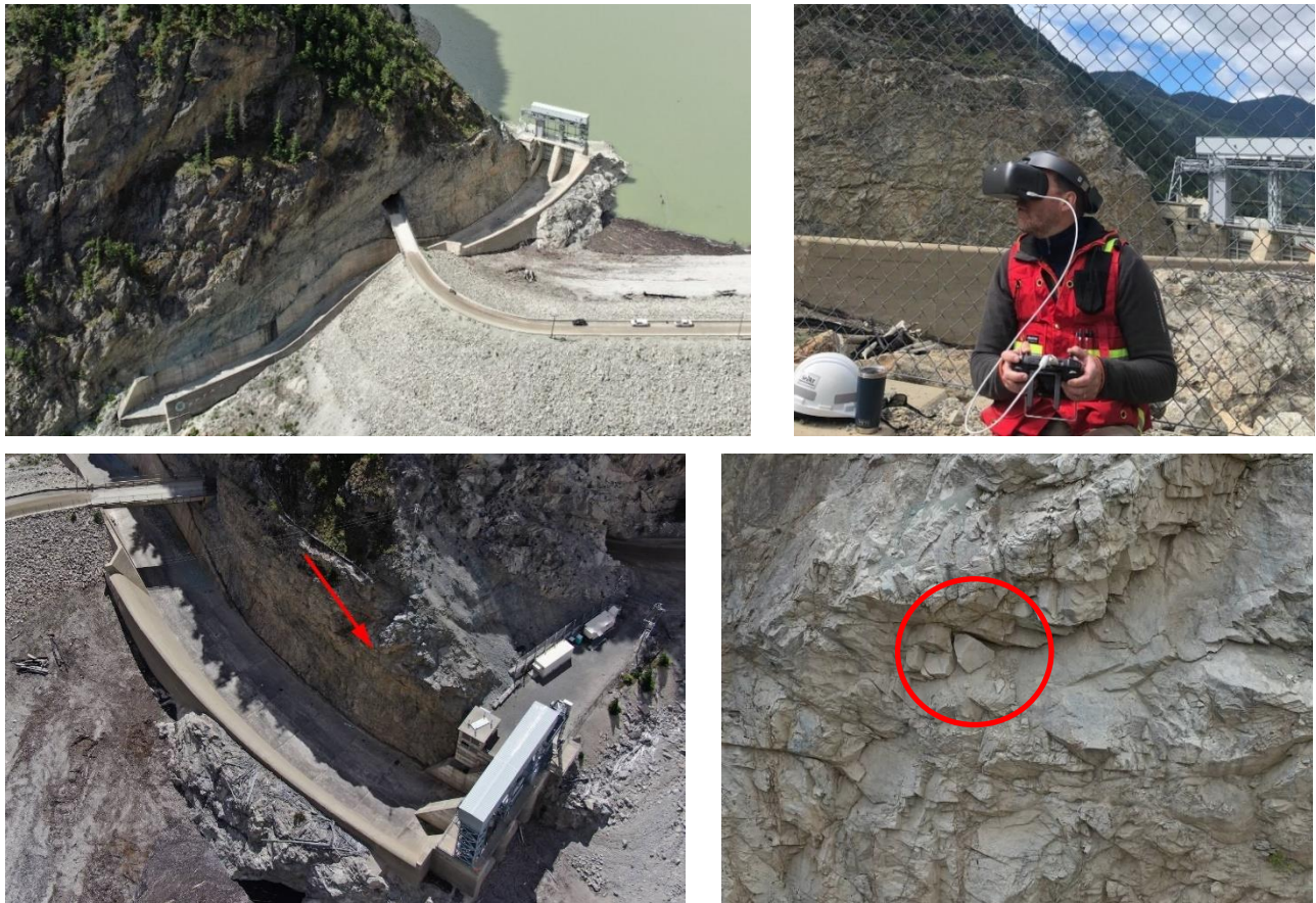
Figure 11 Terzaghi Dam spillway chute rock wall inspection. Overview (top left), engineer controlling the drone's high resolution camera (top right), location of a loose, hazardous rock (bottom left), and close-up view of the hazardous rock which is approximately 0.6 metres or 2 feet wide (bottom right).
