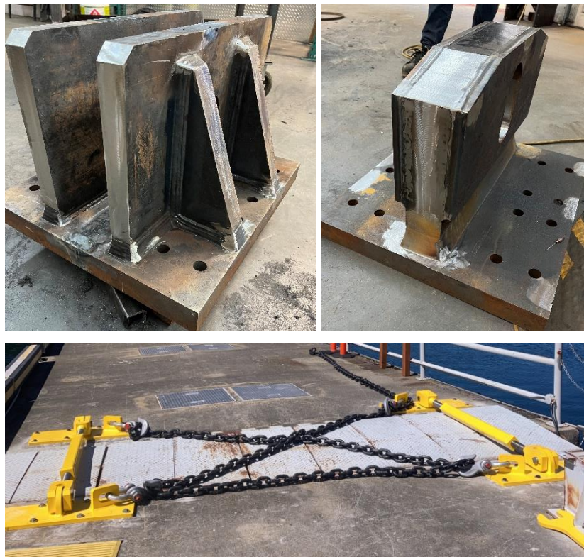
Figure 4 Fabricated replacement hinge components (top) and installed bracing frame (bottom).
