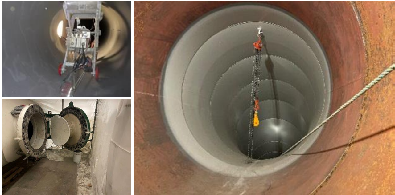
Figure 9 Recoating of the Bridge River 2 Penstock 2. Top left: coating robot inside the penstock. Bottom left: New access hatch installed by the project. Right: penstock before (foreground) and after (background) recoating.
