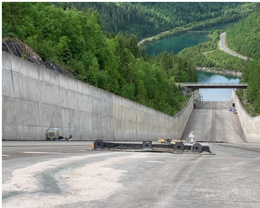
Figure 5 The Mica Dam spillway with repairs to the centerline crack underway.
