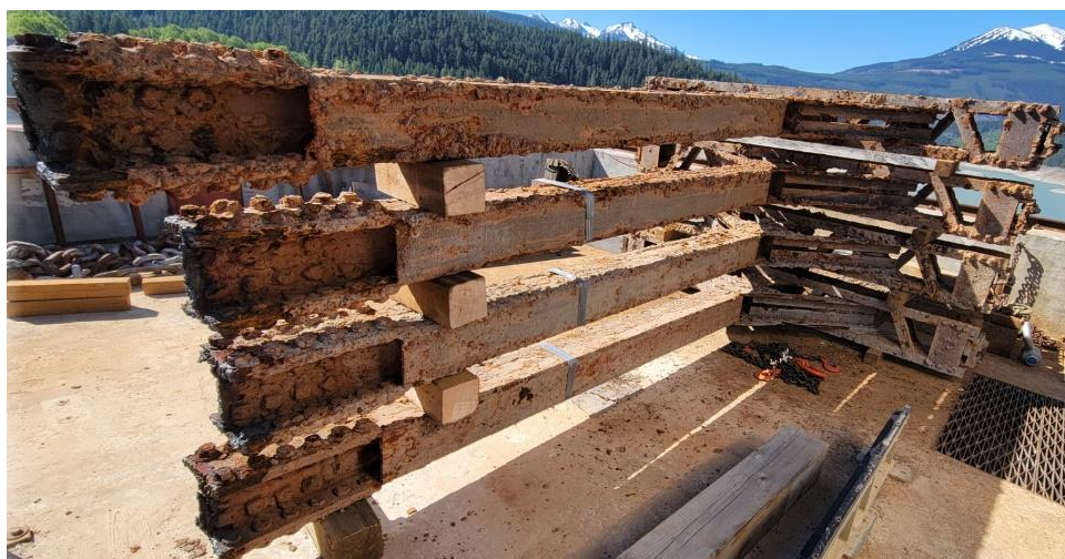
Figure 9 Replacement of Intake Operating Gate 3 cruciform followers at La Joie Dam. Heavily corroded followers that were removed are shown above; newly fabricated and installed followers at right.
