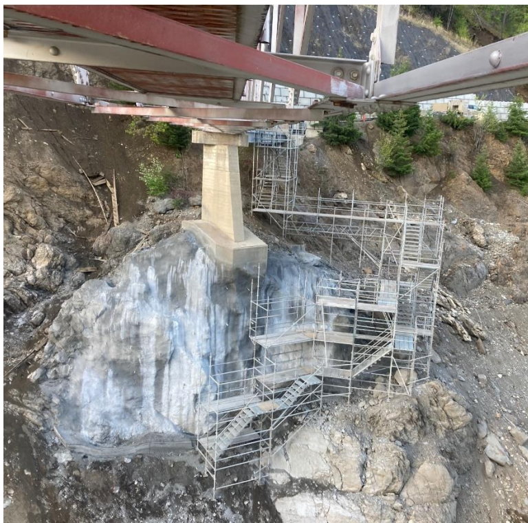
Figure 7 Stabilization of a bridge pier at the Bridge River 2 Generating Station intake tower.
