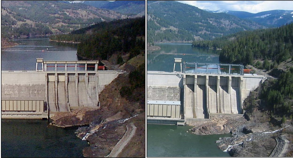
Concrete gate towers and hoist house structure (left) were replaced with steel towers and five hoist housings at deck level in 2005 (right)
