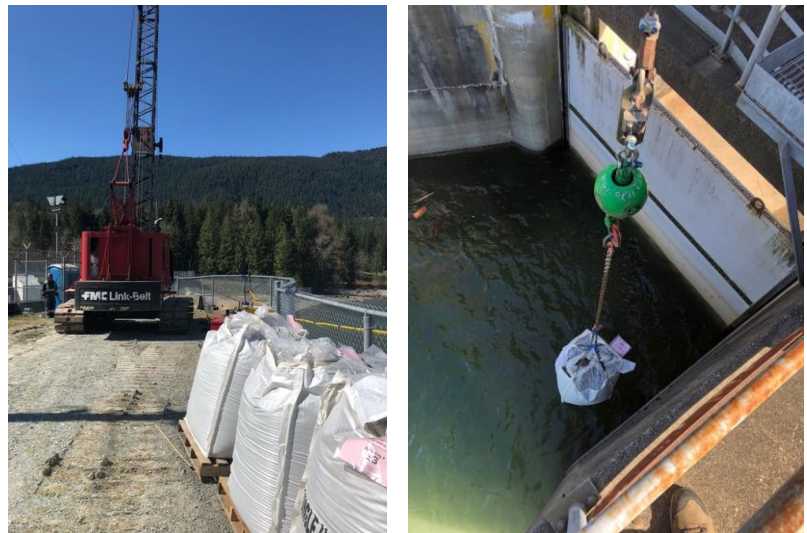
Figure 1 Left: staging of crane and Superbags on the crest of Alouette Dam. Right: test placement of Superbag upstream of the sluice gate.
