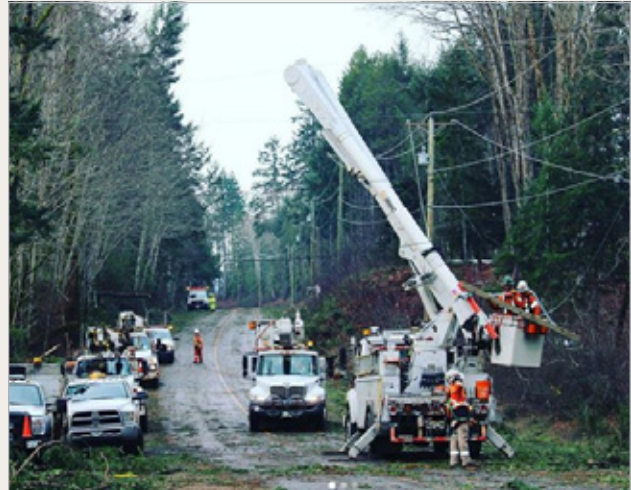
Figure 16: Crews responding to downed lines, December 2018
