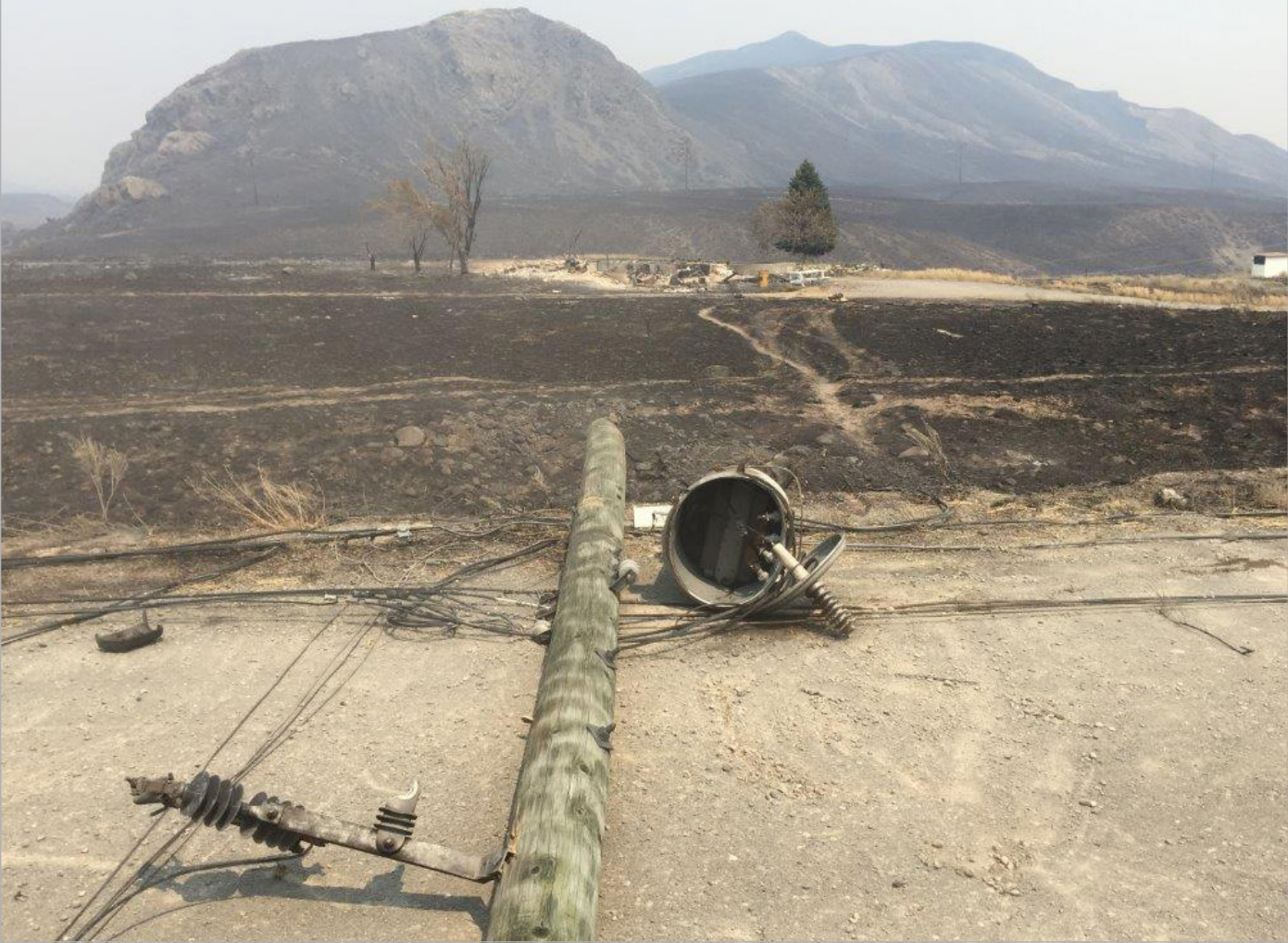
Figure 9: A power pole burned down by the 2017 wildfires
