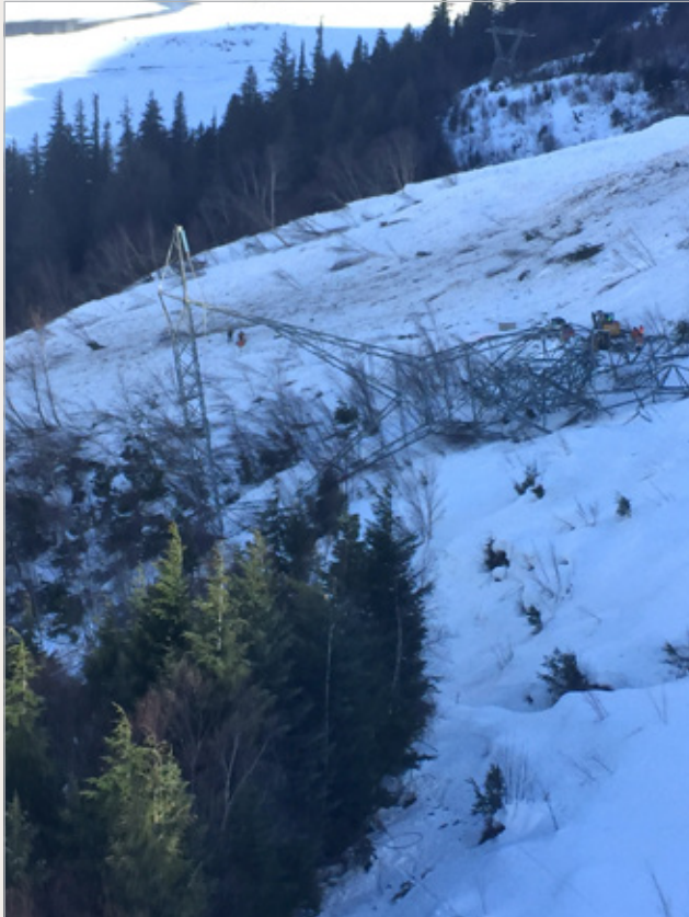
Figure 14: The damaged tower, March 2018
