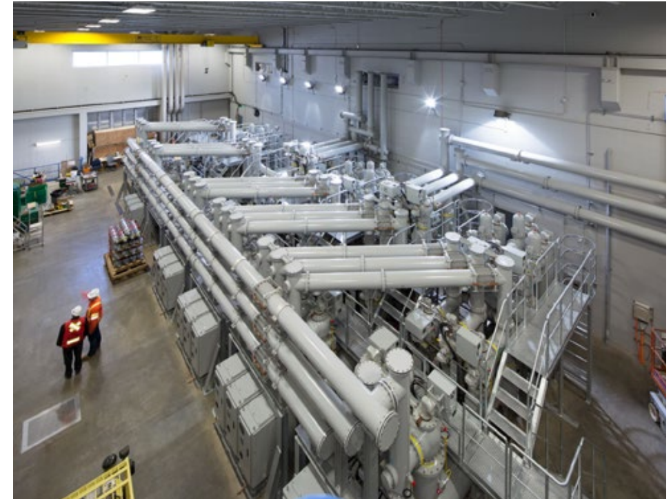
Inside the Mount Pleasant substation
