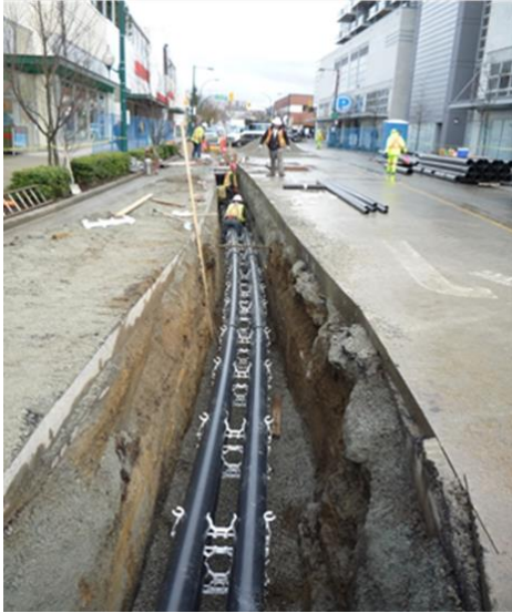
An example of duct bank construction and underground cable.
