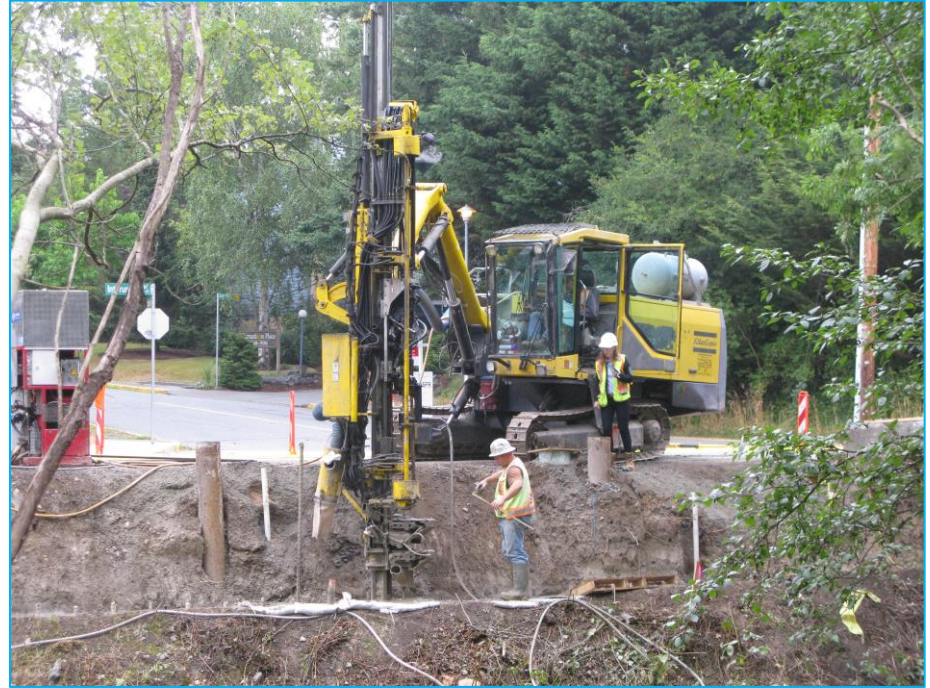
Photos from 2013: Soil remediation work to remove mineral oil beside Colquitz Creek. The work also included bank stabilization.
