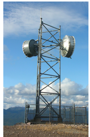
Communications tower example
