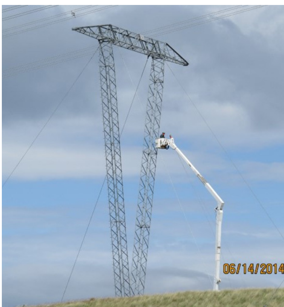
Lattice Guyed Flat Tangent (most PGGT towers)
