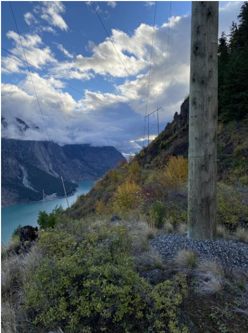
Transmission line 2L90 overlooking Seton Lake
