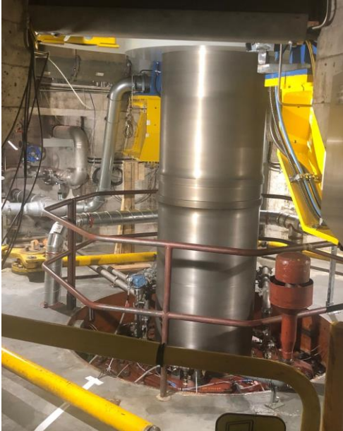
The newly commissioned Unit 7 generator at Bridge 2
