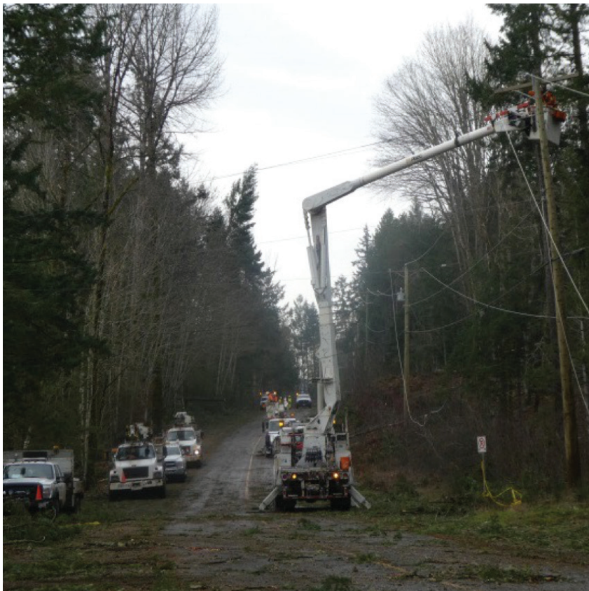
Crews repairing extensive damage in Nanaimo following the December 2018 windstorm, the most destructive in BC Hydro's history.
