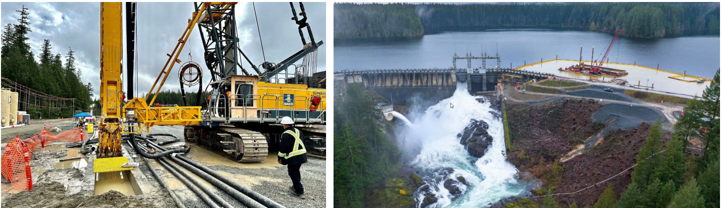
Figure 8 Construction on the John Hart Dam Seismic Upgrade Project. Left: Construction of a panel of the plastic concrete cut-off wall, showing the specialized excavating equipment in use (November 2023). Right: Looking upstream toward the North Earthfill Dam work site (January 2024).
