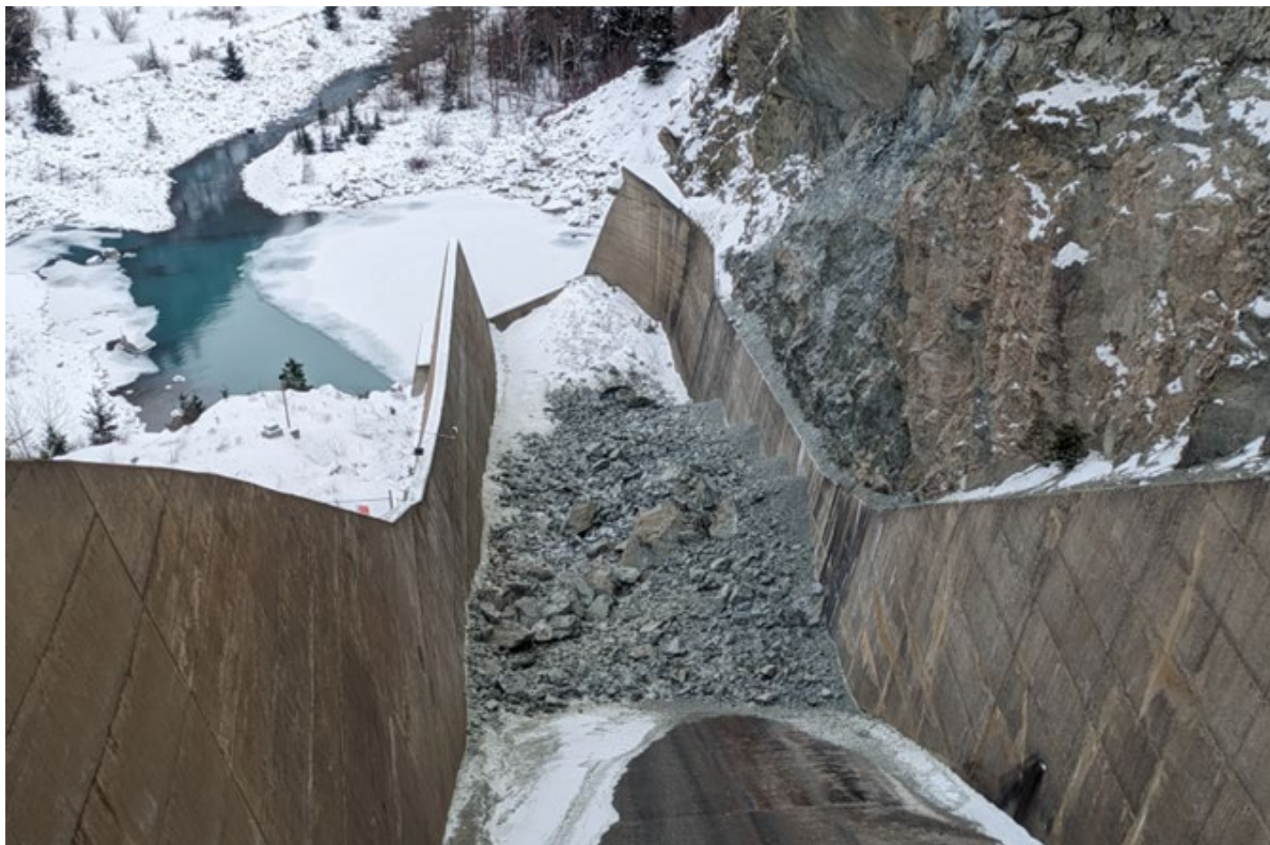
Figure 4 Rockfall in the spillway at Terzaghi Dam.
