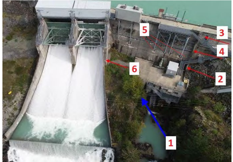
Figure 4 Drone photo showing areas of Cheakamus Dam where concrete is deteriorating due to alkali aggregate reactivity.
