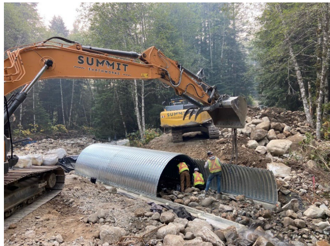
Figure 8 Installation of a new culvert under the Wahleach Dam access road to prevent future washout.
