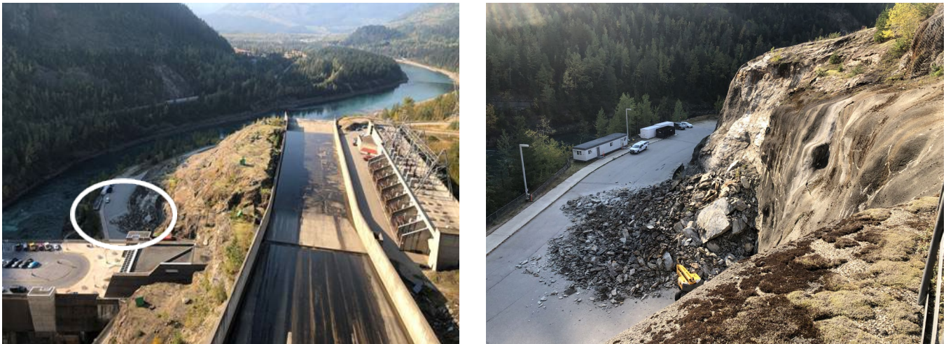
Figure 3 Rockfall on the Marble Shear Block at Revelstoke Dam and Generating Station. At left: the location of the rockfall as viewed from above the spillway. At right: view of the rockfall onto the access road and main parking lot of the generating station.
