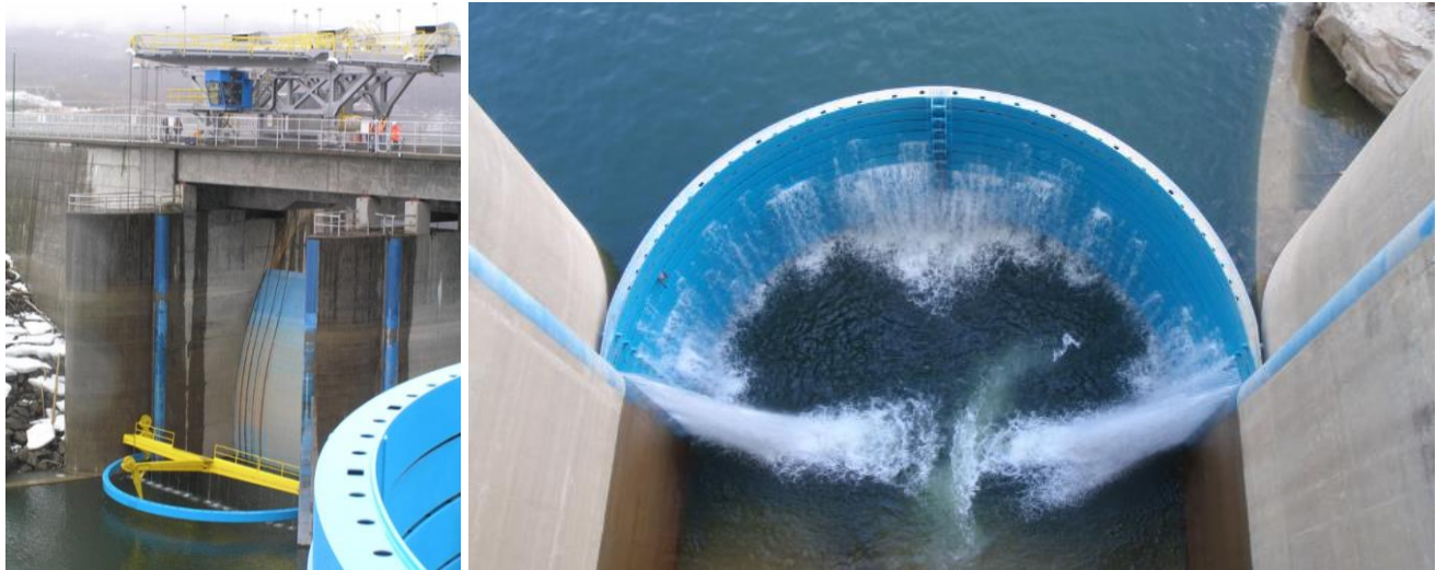
Figure 10 At left: a spillway stoplog (blue semi-circular object) being installed at WAC Bennett Dam. At right: excessive leakage through the existing stoplogs as viewed from above.
