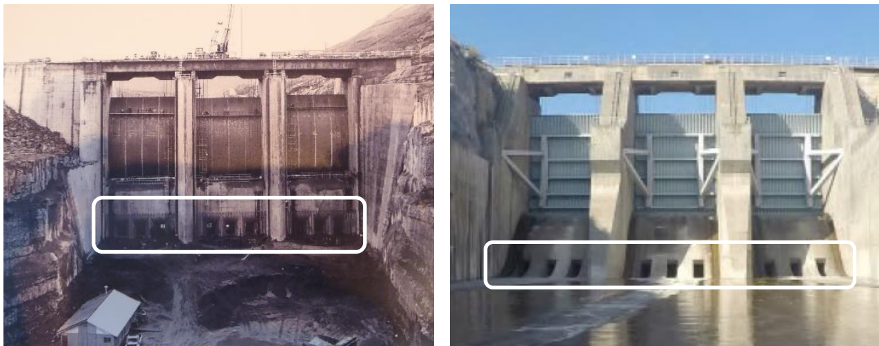
Figure 9 Sluiceways (outlined) on the spillway of WAC Bennett Dam, as viewed from upstream during construction (at left) and from downstream on the spillway chute (at right).
