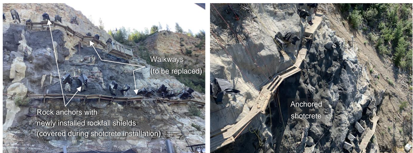
Figure 8 Slope stabilization work completed on the 731 Block on the rock slope above Revelstoke Generating Station, as seen from Highway 23 (left) and from above (right).
