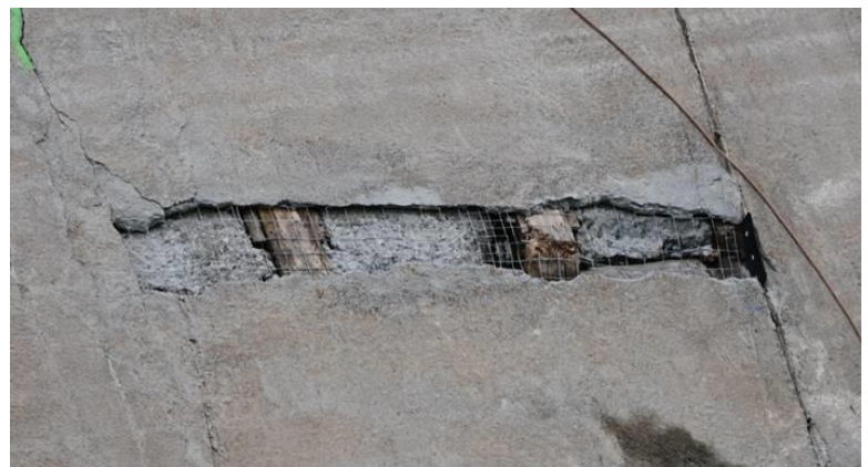
Figure 7 Large repair area chipped open and exposed at the lower portion of Panel 70-71 on the face of La Joie Dam.
