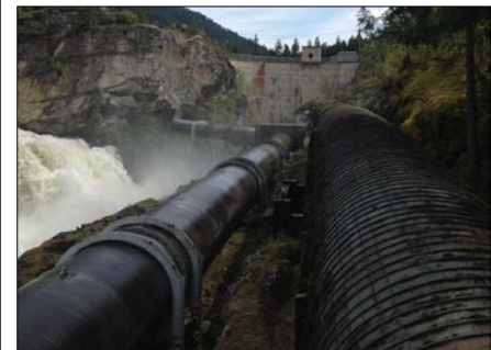
Steel and woodstave penstocks
