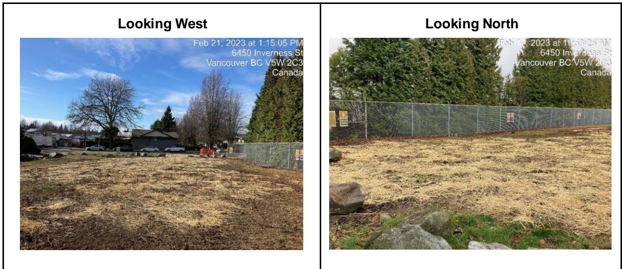
Figure B-4 Disturbed soil covered with straw for erosion and sediment control, south side of the property, February 2023
