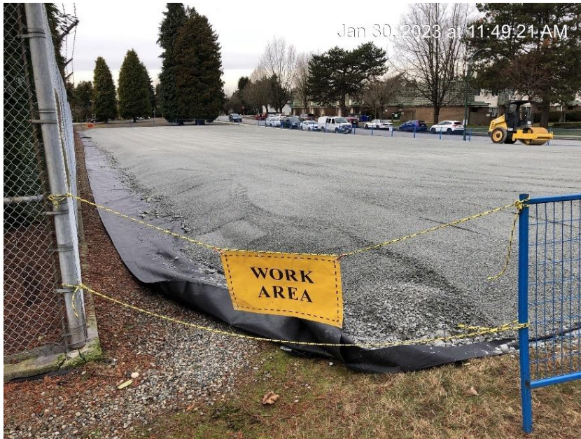
Figure B-2 Temporary parking area constructed on north side of the property, January 2023
