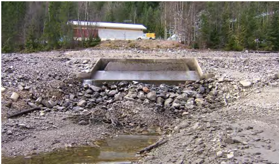
Figure 2. Outlet structure with no turbine outflow. The small amount of discharge from the HVAC system can be seen at the far left of the structure (April 17, 2012). Walter Hardman Generating Station is in the background.
