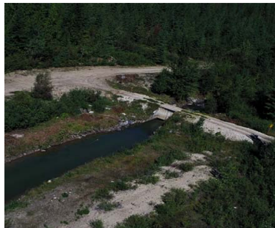
Photo 2-4: Orifice Control Structure (right, downstream of stoplogs and facing downstream in diversion channel)
