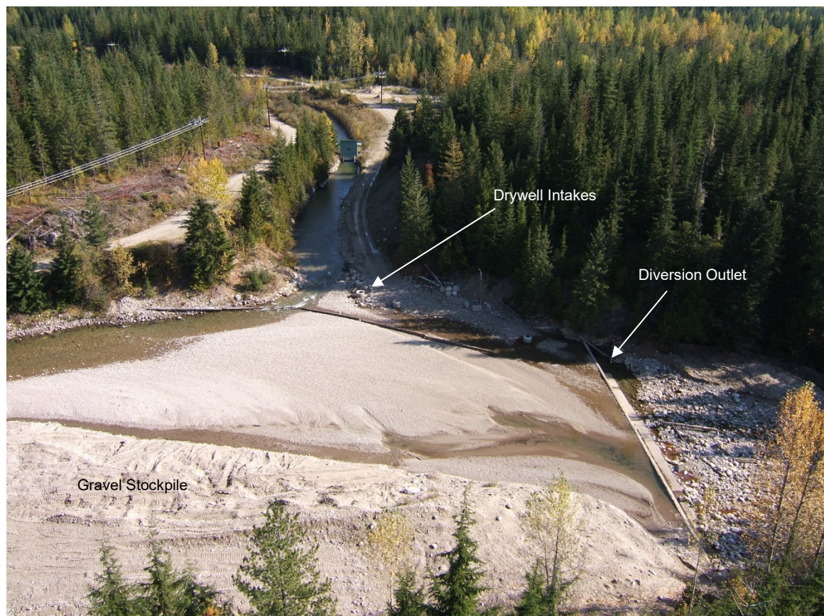
Figure 4.2 Aerial view looking east over the work site, showing the diversion channel, gravel stockpile, drywells (intakes to provide the minimum flow to Cranberry Creek) and diversion dam and minimum flow outlet (October 10, 2008).
